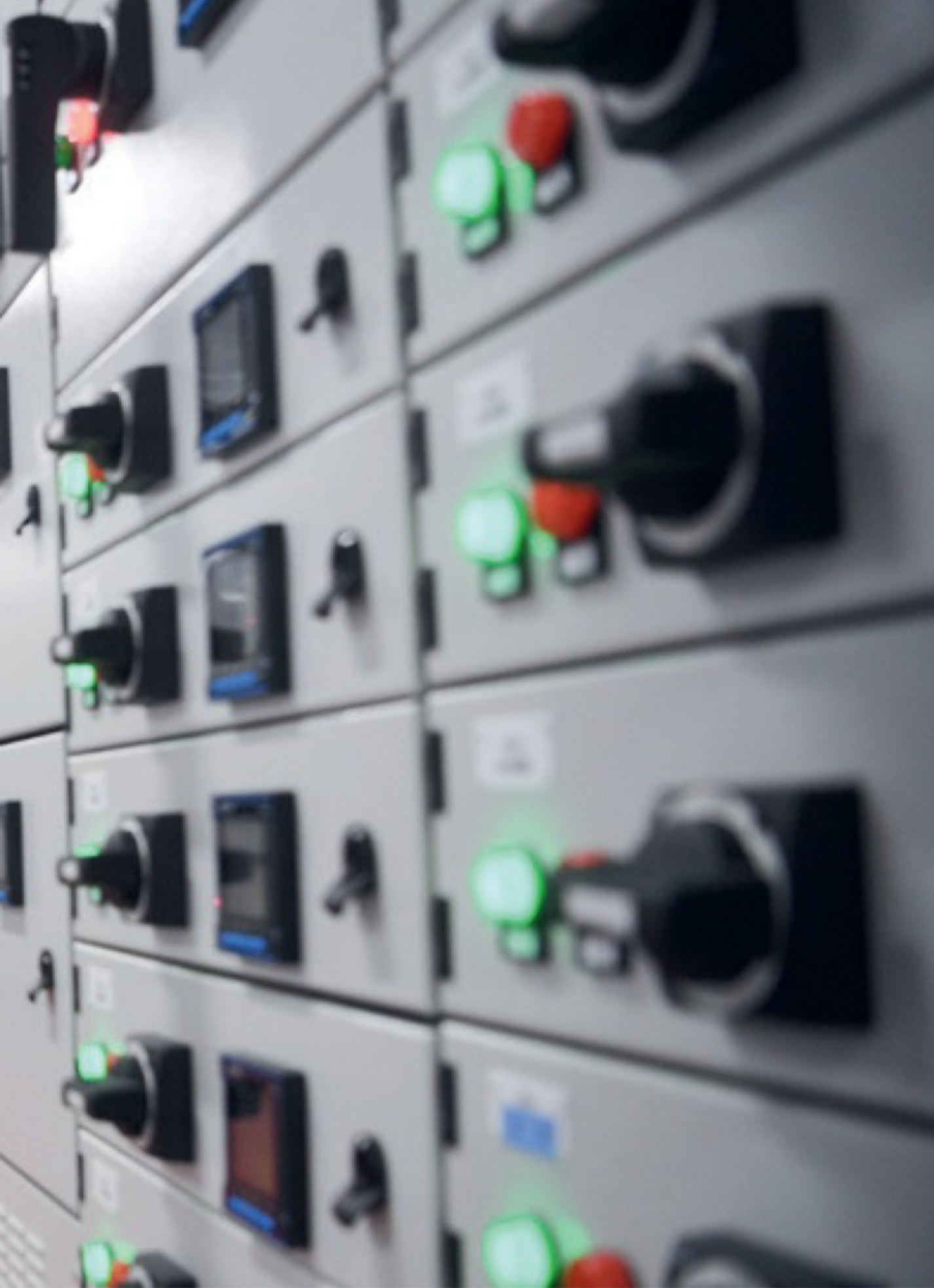
A staff member works at a data center of telecom giant China Unicom in Zhongwei, Ningxia Hui Autonomous Region, on March 1
